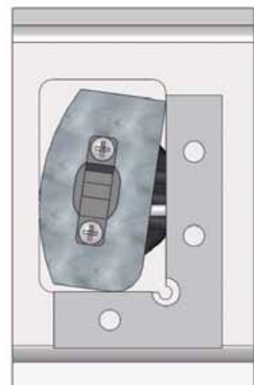
Figure 40: Improper Optical Switch Installation Bottom View 2
